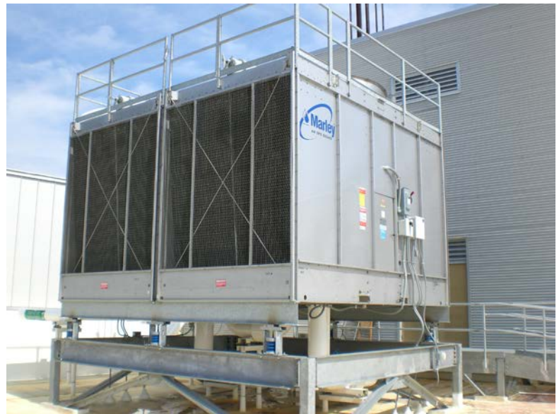
Shown above is an example of a regulated cooling tower
