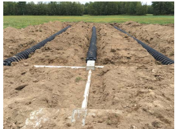
Shown above is an EHS Division inspected infiltration chamber absorption field.
