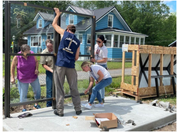
CHSC and St. Joseph's Community Center staff install a new bus shelter at the center.
